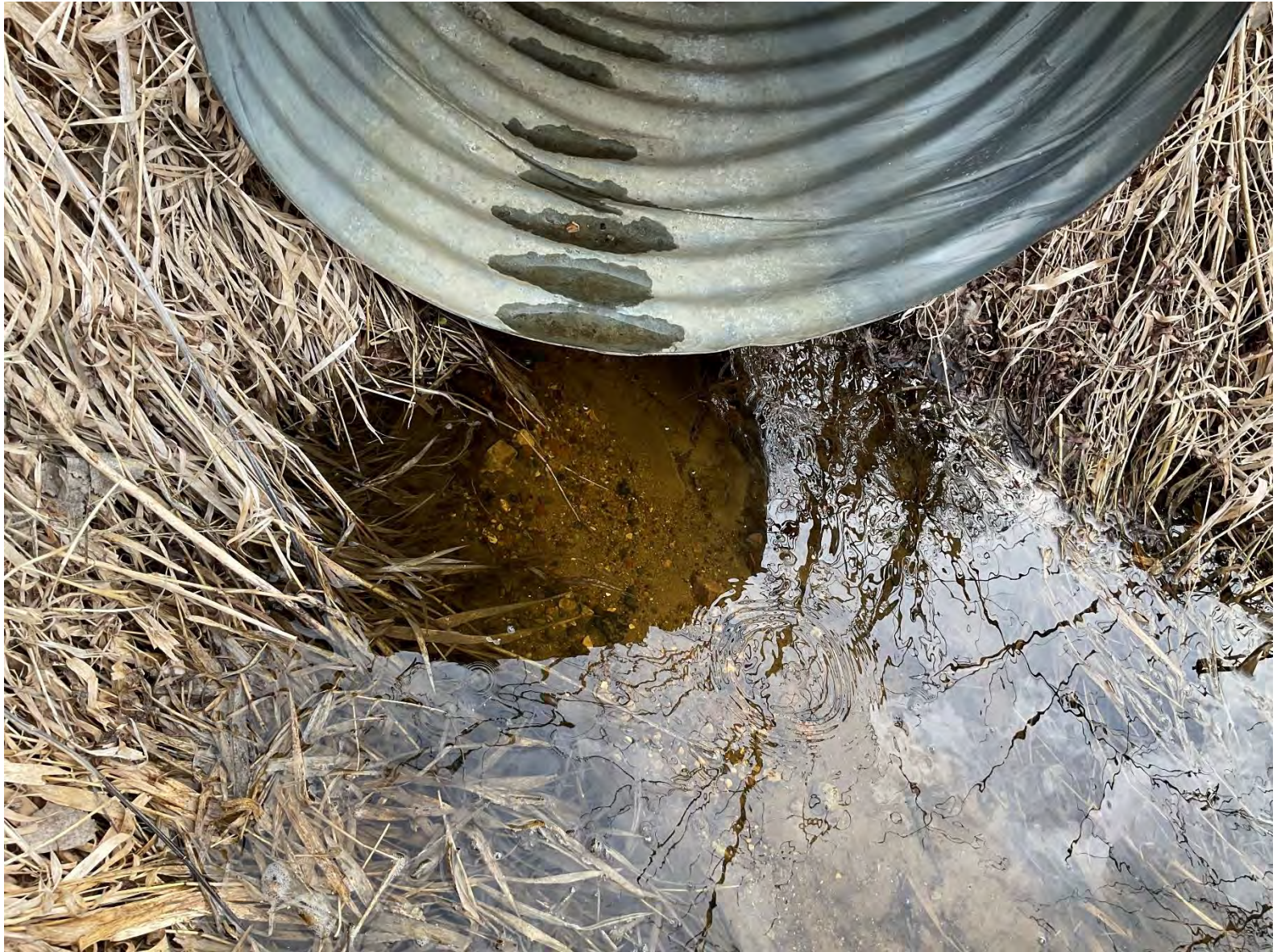
32 – Culvert F Downstream Erosion
