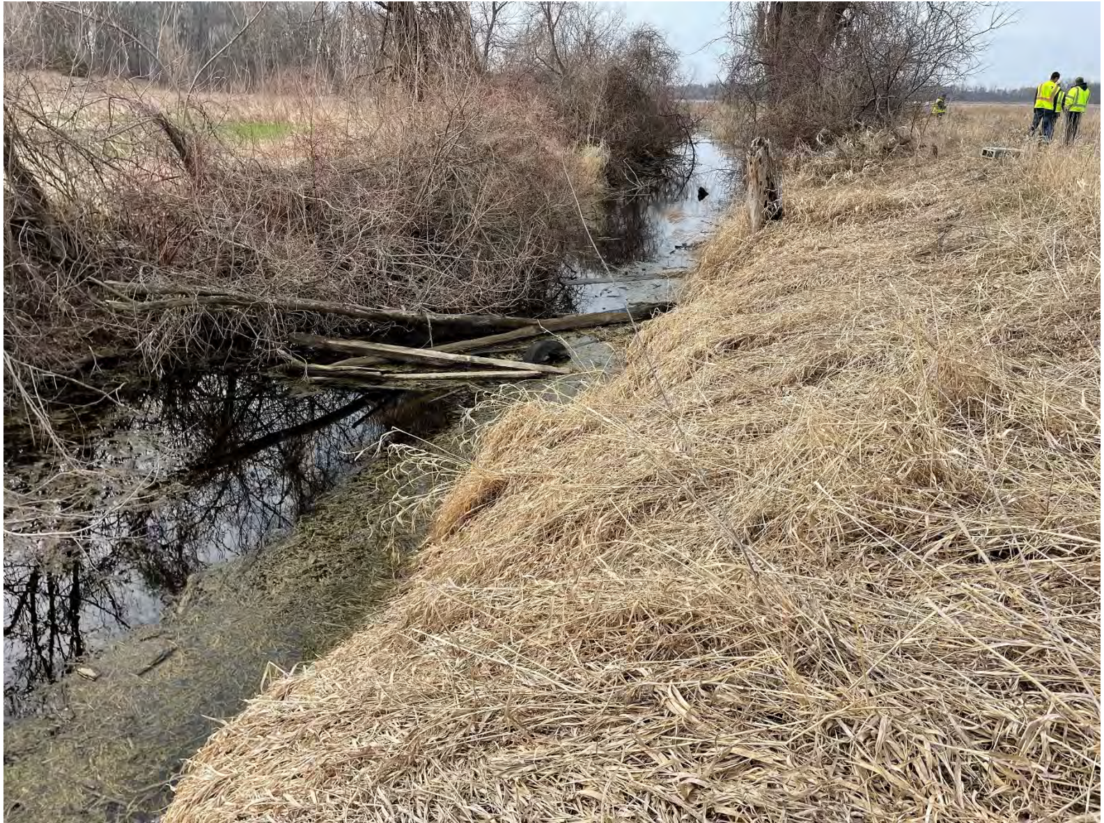
34 – Culvert F Downstream Channel Debris
