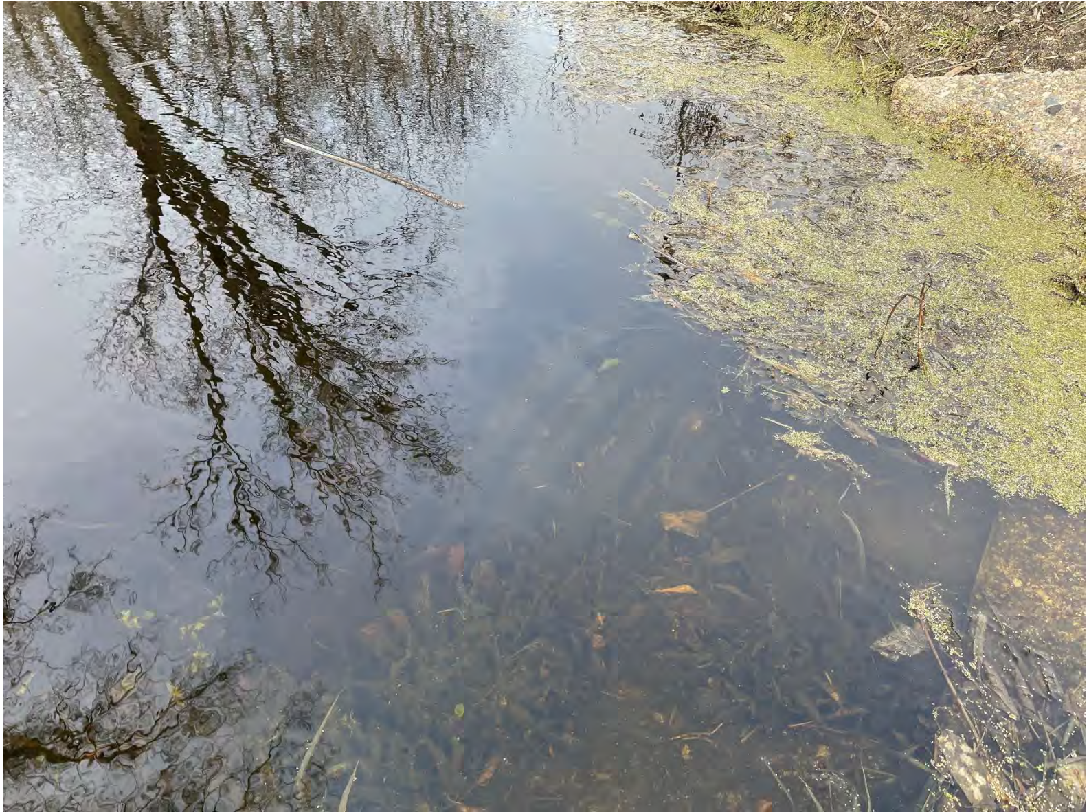
12 –Submerged Downstream End of Culvert D
