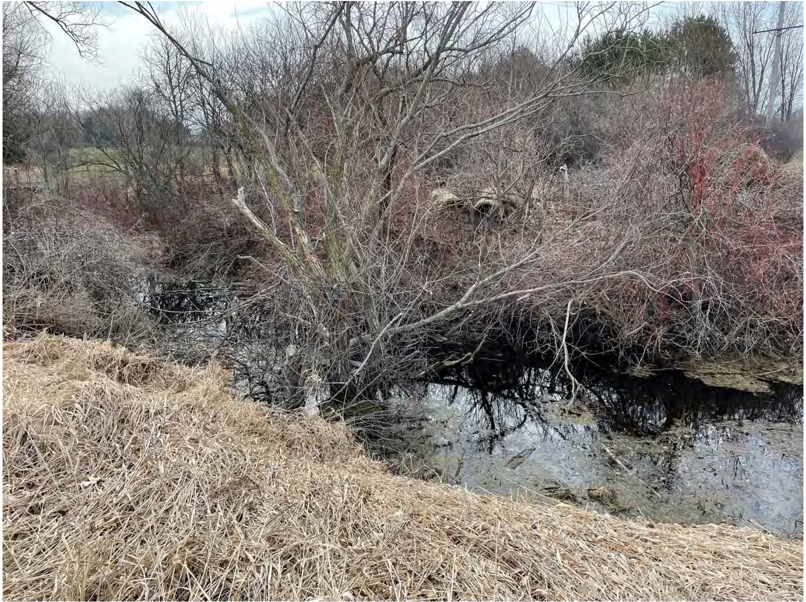
27 – Channel Debris in 1826 Birch St Property
