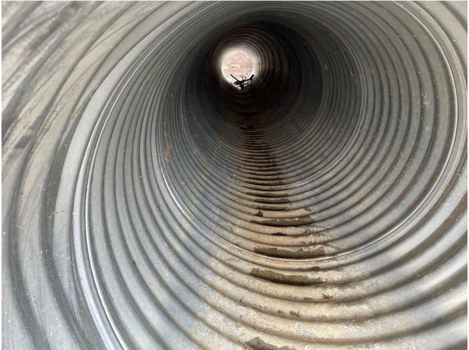
33 – Culvert F Heaving
