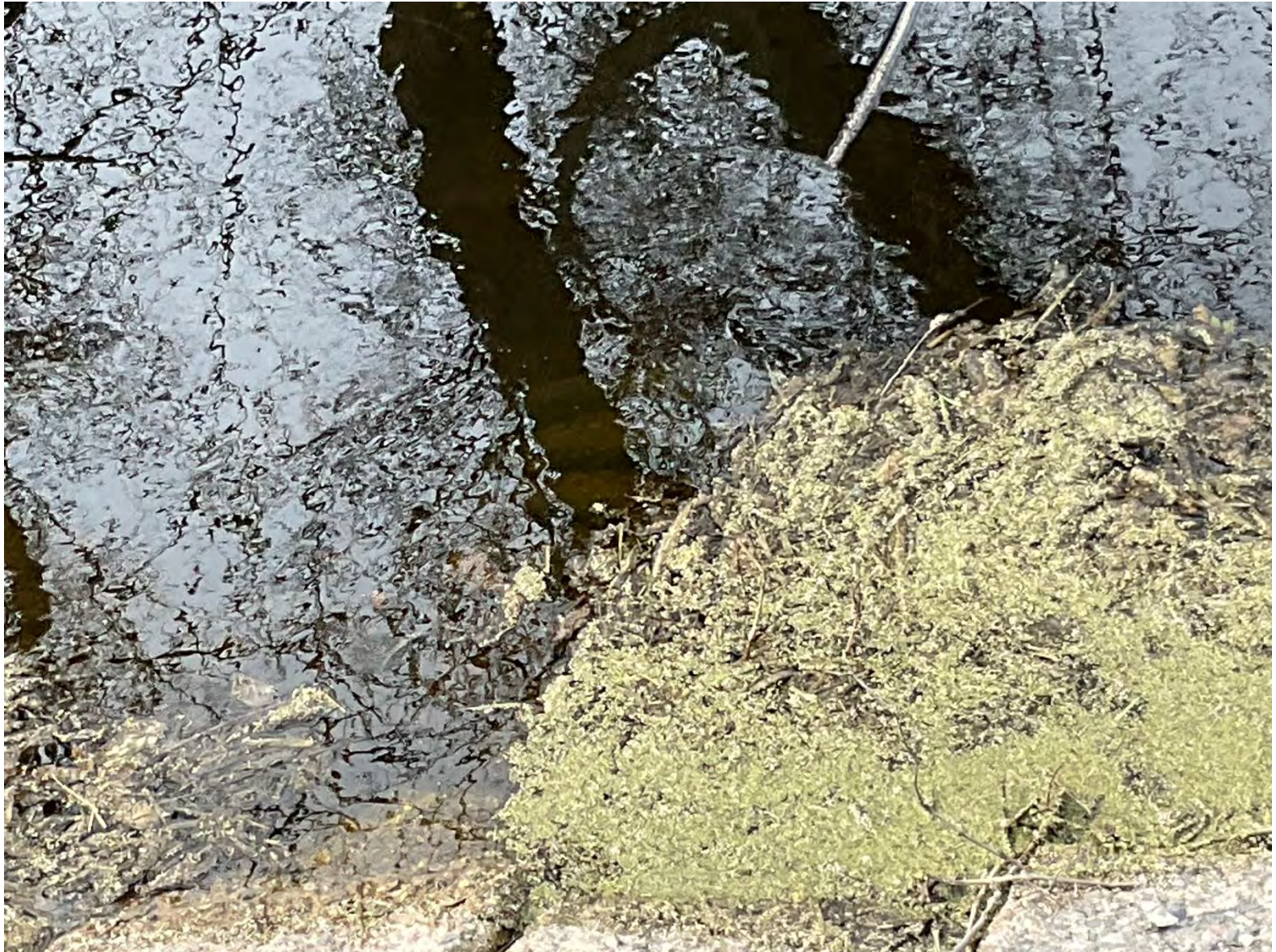
10 –Submerged Upstream End of Culvert D
