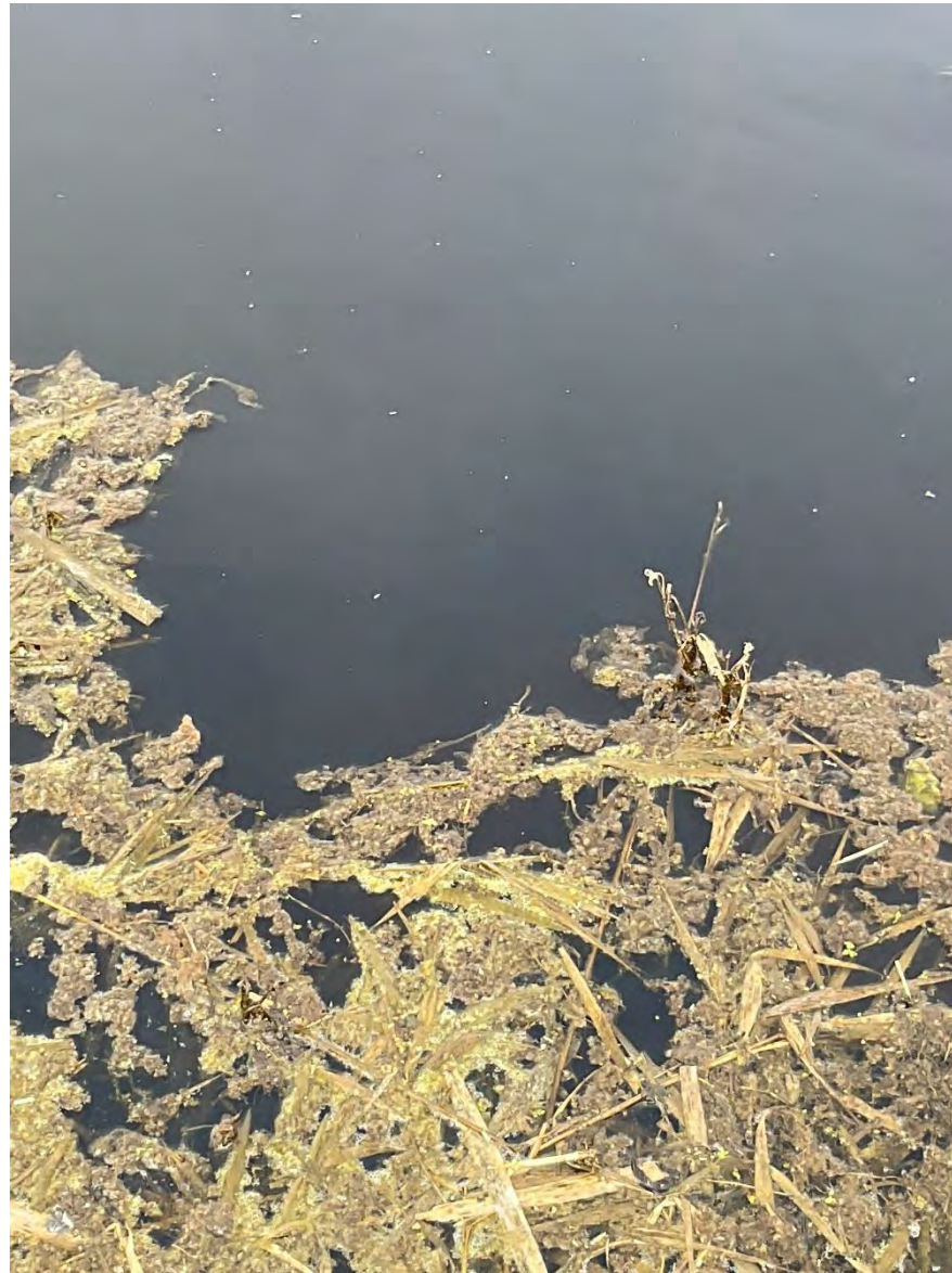
6 – Submerged Downstream End of Culvert C
