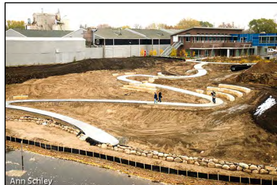
The headquarters before, during, and after construction. Barr provided construction management and oversight services on this project.
