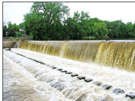
Barr determined that adding new gates along the dam crest and submerged slide gates through each dam bay at the Rum River Dam in Anoka would be the most practical method to prevent the migration of Asian carp.
