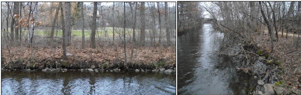
Figure 17. Erosion on the Charley-Pleasant channel, just east of W Pleasant Lake Rd.
